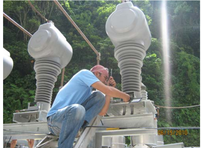
POWERHOUSE A TRANSFORMER
